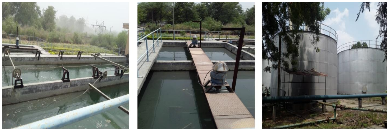
Fig.: the rapid mixing tank, the settling tank and the storage tank of ETP respectively.
