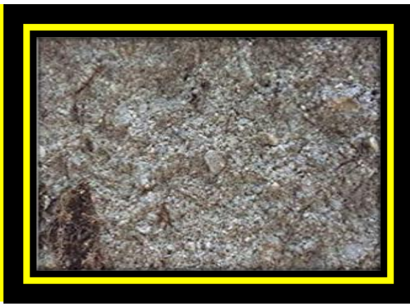
Figure 1 Rough surface of heat exchanger
