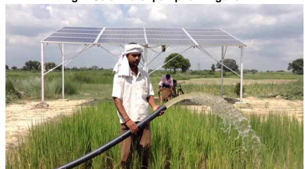
Fig 4. Solar water pump for irrigation
