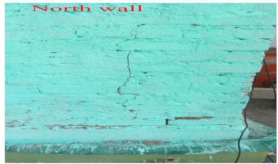
Figure 7 Crack on north wall
