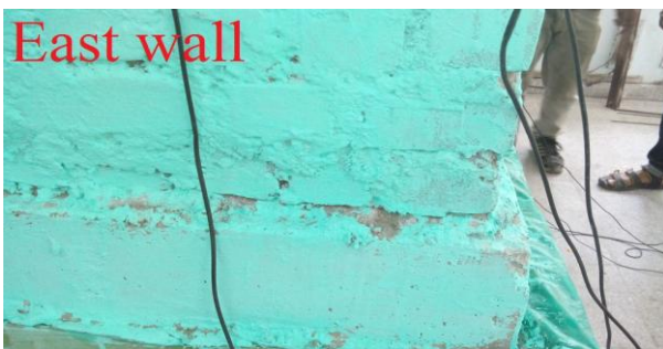
Figure 6 Crack on east wall at base level
