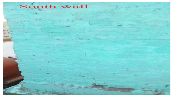
Figure 8 Crack on south wall
