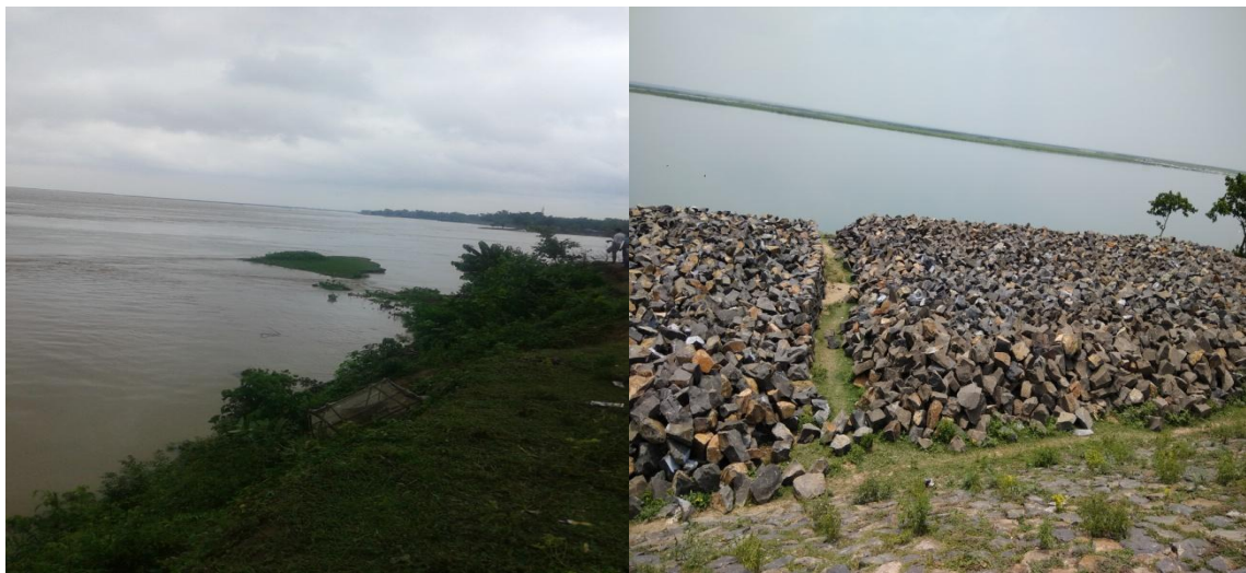
Fig.5 River Bank Erosion at Palgachhi & 6. Revetment at Palgachhi Mouza
